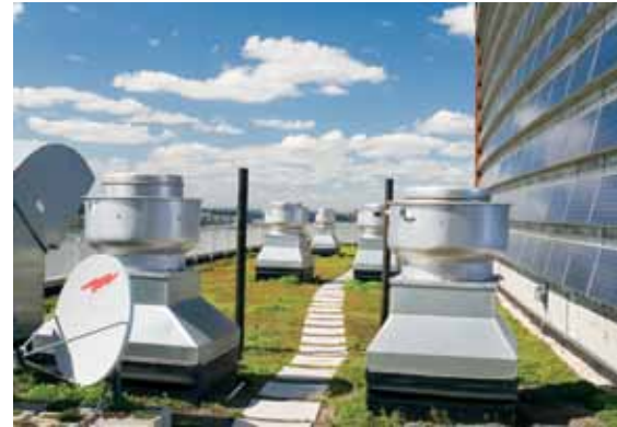
Greenheck exhaust fans on roof of Solaire.
