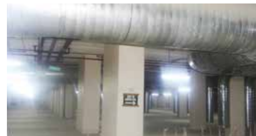
Camellias' basement ventilation.
