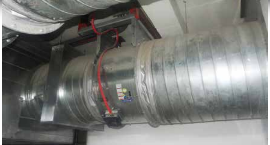
Greenheck's Model RA axial fan in the underground parking area.
